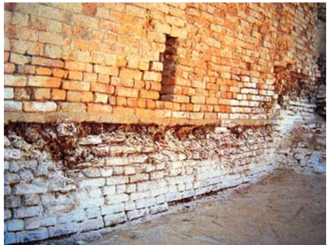
A mud-brick wall in the lower town of the Indus center Mohenjo-daro shows signs of severe salt damage.
