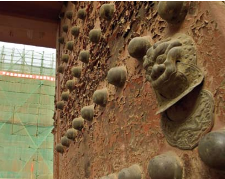
Paint peels from a 10-foot wooden door near the north entrance to the Forbidden City, a common problem at the imperial complex where exterior surfaces are exposed to direct sunlight and city pollution.
